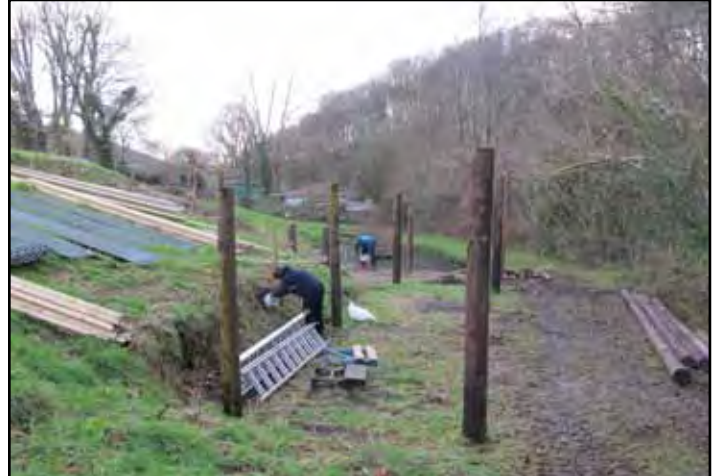
Richard and Leigh-Anne Boucher worked with our Head of Conservation David for five days in wet, cold and extremely muddy conditions. By Thursday afternoon they were up on the roof.
